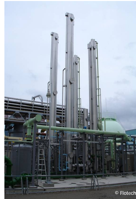
Flotech CSFR-225, Higashinada, JP
